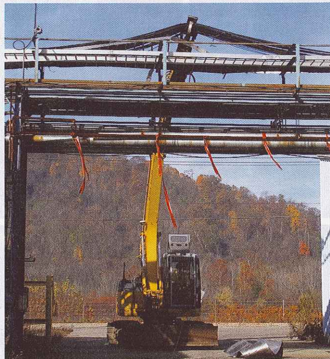
The enhanced visibility provided by the MT's streamlined design allows Eslich to surgically remove copper lines from each section of the plant with the MTR 15 S.
