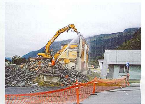
The MTR 20 is used to demolish an old hospital structure standing very close to the new hospital wing.
