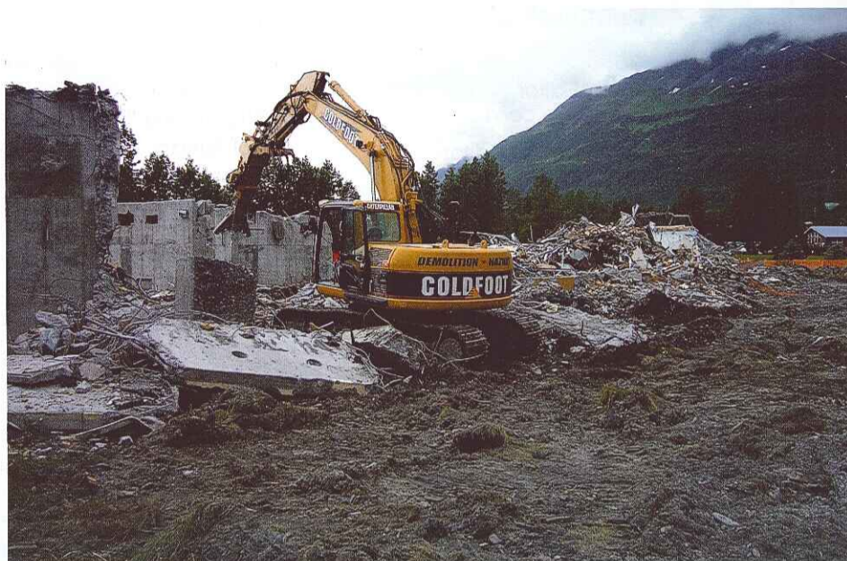
The MT 20 Cracker/Crusher Jaw Set is used to process and de-rod over 11,500 cubic yards of concrete.
