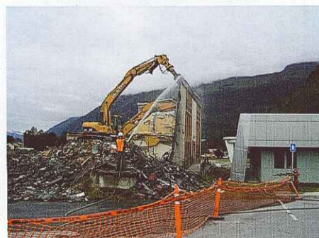
Coldfoot Environmental used the MT Series Multi-Tool model MTR 20 to demolish an old hospital structure standing in very close proximity to the new hospital wing.
