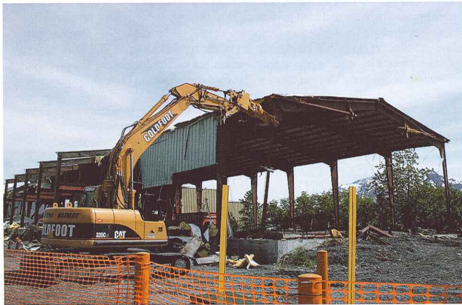
An Allied-Gator MTR 20 with a Shear Jaw Set enabled Coldfoot Environmental to demolish this former fish processing plant quickly and efficiently, finishing the project substantially ahead of schedule.
