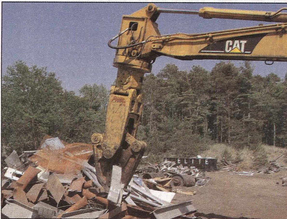
"Pitsch Enterprises utilizes the Allied-Gator MTR 70 S to quickly and effectively process the project's heaviest scrap materials."
