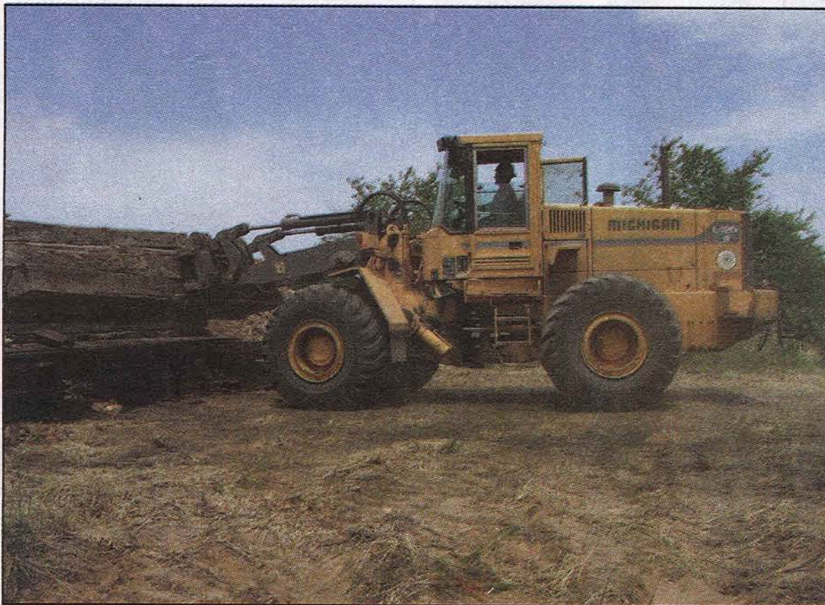
Mark Mushong hauls old crane mats to the grinding work area, operating a Volvo L120 wheel loader equipped with a Volvo fork attachment.
