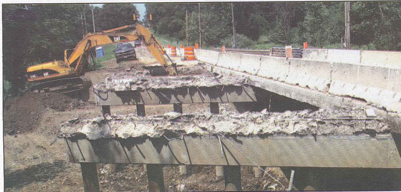
B.O.G. finishes demolition on the first bridge lane in less than one day and must immediately reconstruct the bridge decking on the existing piers and columns.
