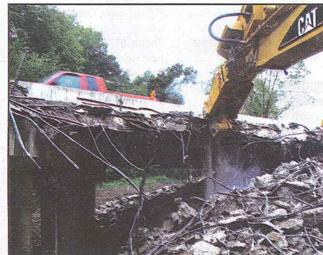
One lane of the Conotton Creek Bridge had to remain open at all times, and safety of passing traffic was the highest priority.
