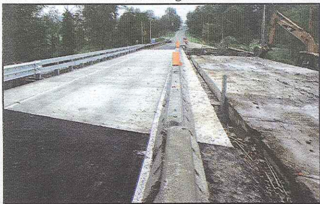
As soon as the first bridge lane was reconstructed and ready to handle traffic, demolition on the second lane began.
