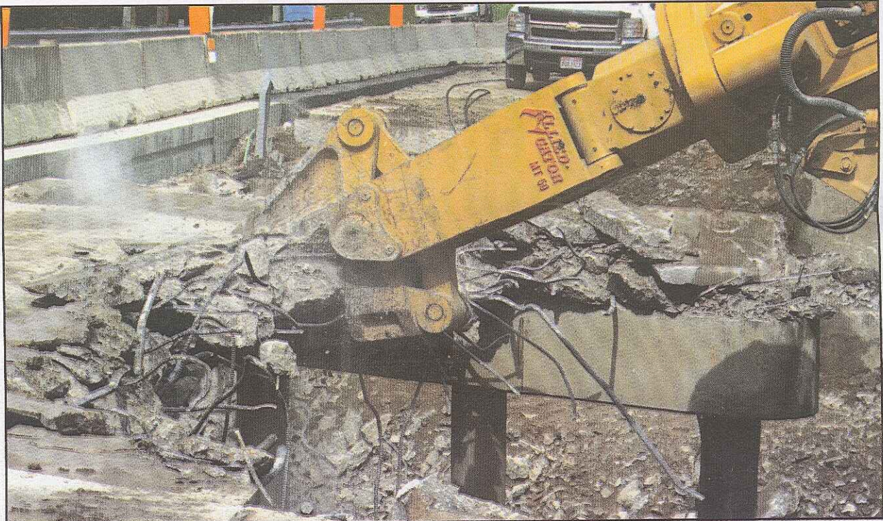
The Allied-Gator MTR 50 C finishes demolition of the second lane of the Conotton Creek Bridge decking in six hours.
